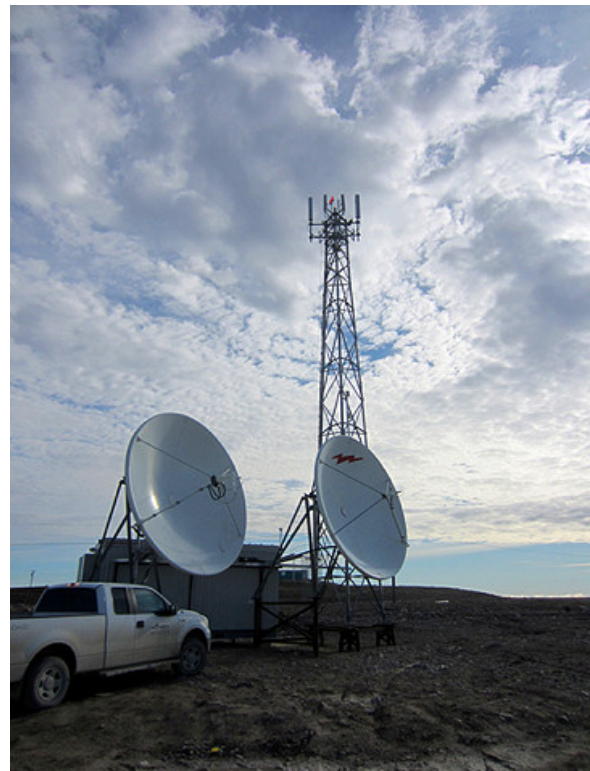
SSi Micro dishes and tower in Cambridge Bay. The federal government recently announced the company will receive $35 million for improving Internet services in Nunavut. - photo courtesy of SSI Micro
